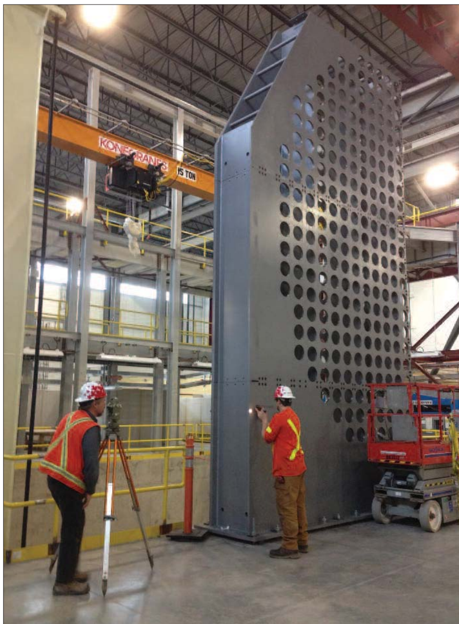
Millwrights leveling a section of a full-scale reactor mock-up of a Darlington reactor inside OPG's new state-of-the-art training facility located in the Darlington Energy Complex.
